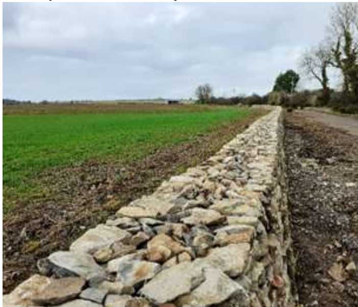
Part of the drystone wall at Tynings, being restored through the Farming in Protected Landscapes programme
